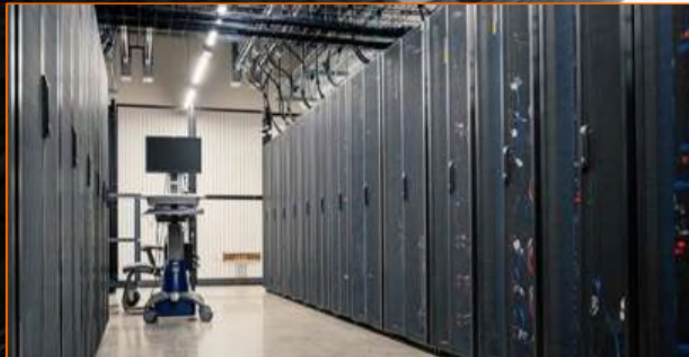
Data Centre & Banking
